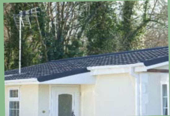
A close-up of the new Decra roof, which comes complete with an impressive 40-year guarantee
